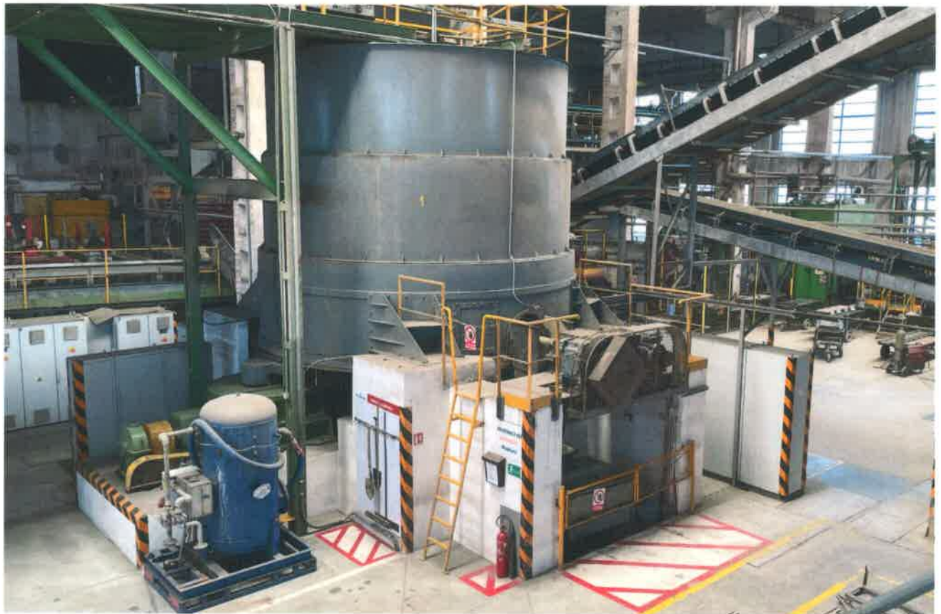
2 | Production mixture silo
